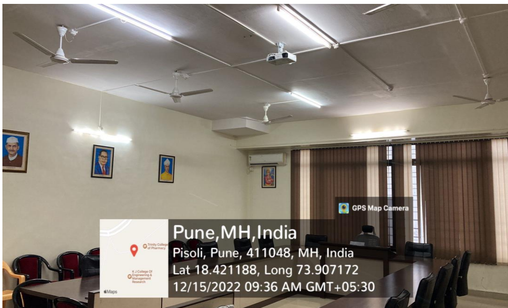
LED lights in board room
