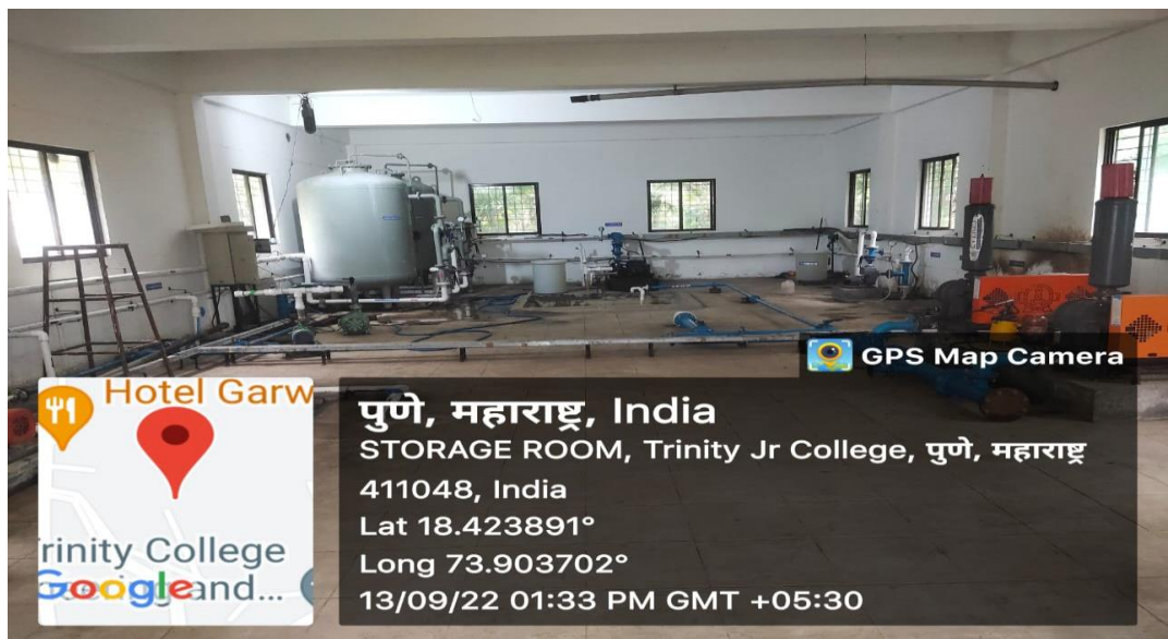
Sewage Treatment Plant (STP)
