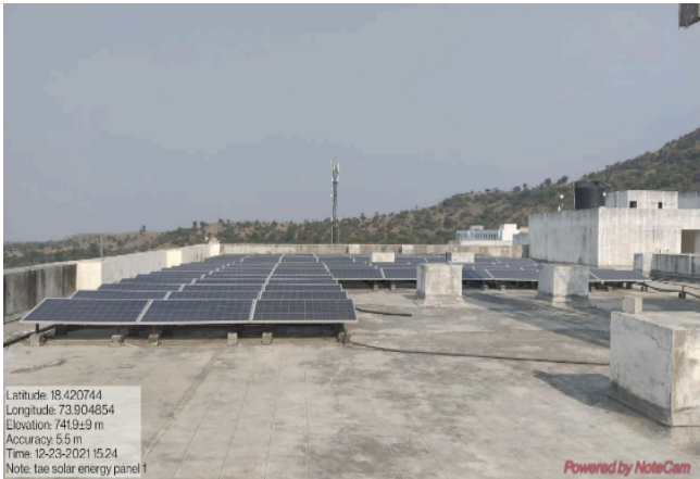
Rooftop Solar System
