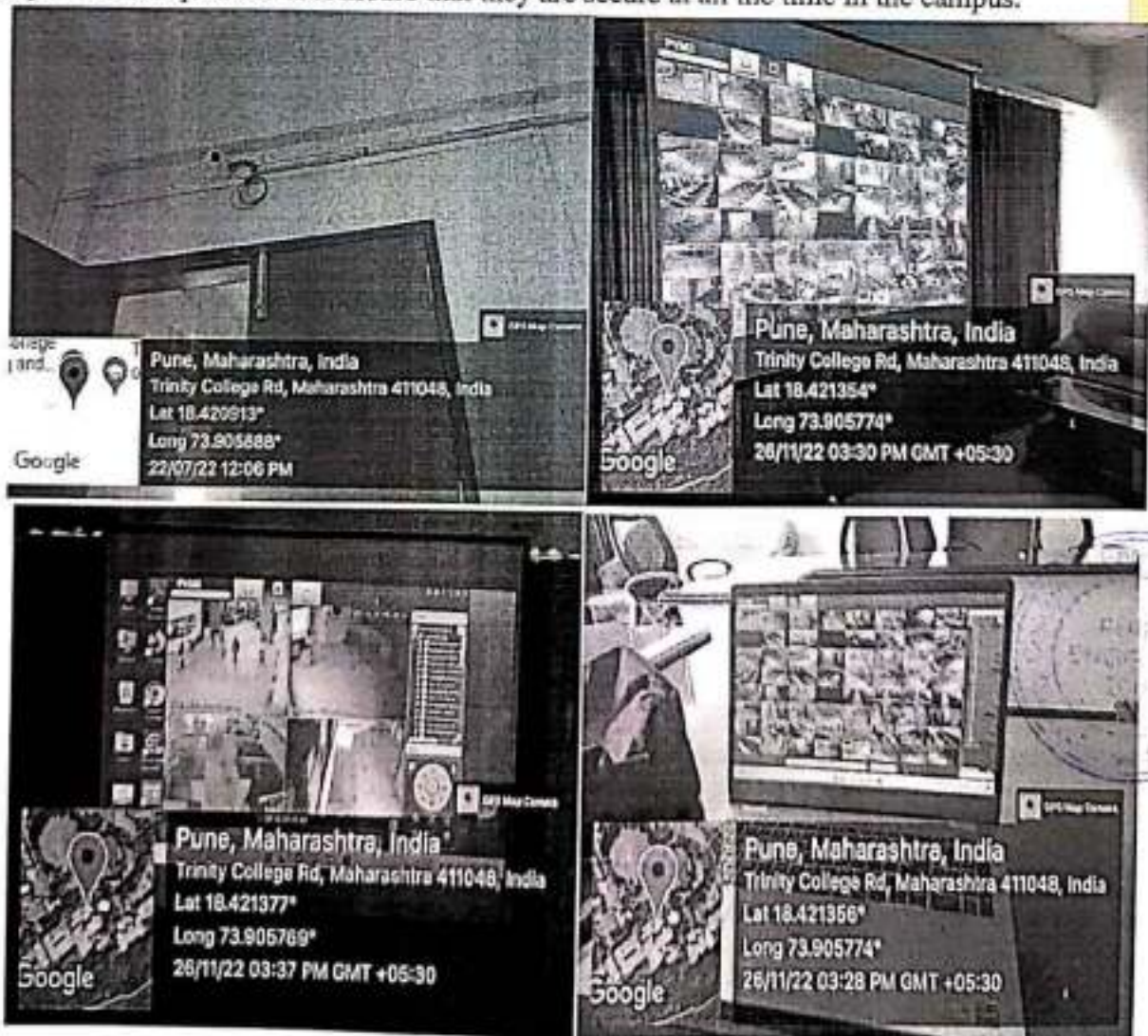
Fig. Surveillance System at Each Room of the institute.
